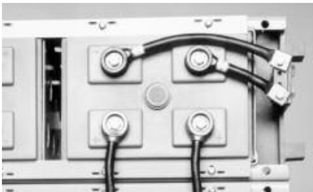
Figure 8: Take-off connectors between cell terminal and main terminal plate
